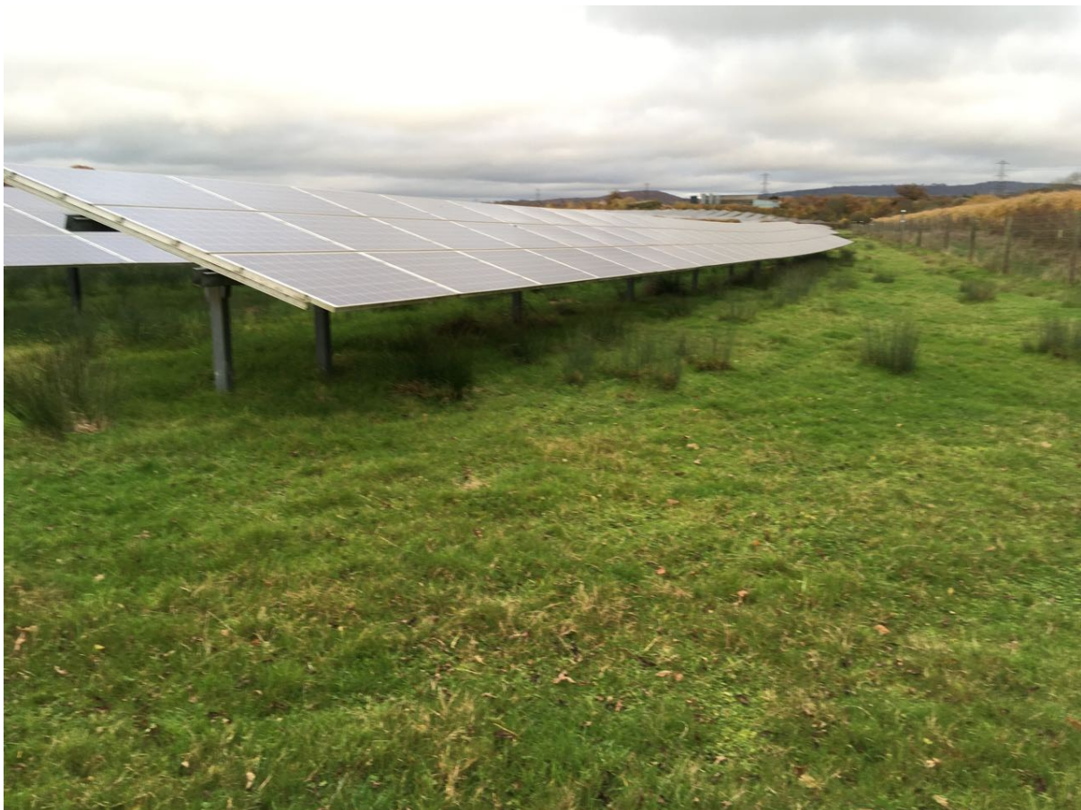
Figure 6-1 Drainage of solar panels onto grass
